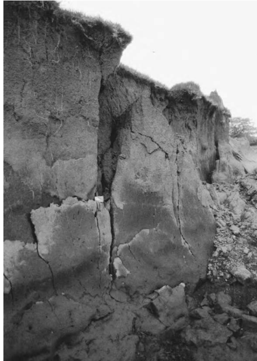
Plate 7.3 Slab failures in cohesive banks, River Ure, North Yorkshire, England.
